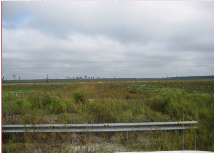
THSF Figure 3: Road removal as part of the Doyle Creek Restoration Project, implemented through NFWFMD with FDOT mitigation funds.
