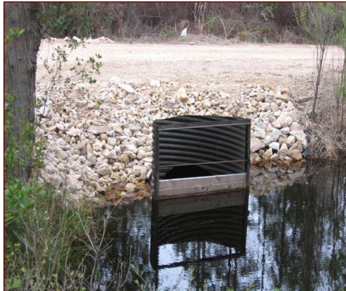
THSF Figure 1: A flashboard riser on John Allen Road allows water level manipulation during the year to accommodate forest management activities.
