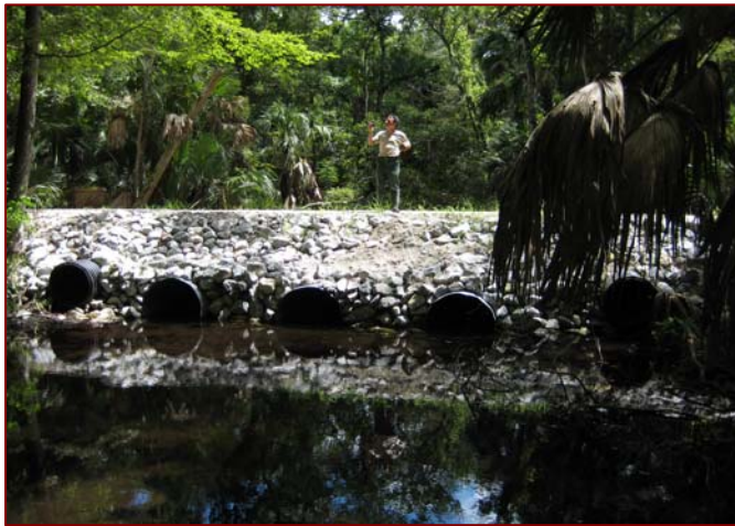
SSF Figure 2: Improved culverted crossing over Sulphur Run on Palatka Road on the Seminole Tract.
