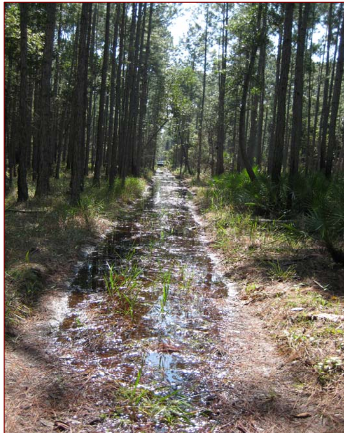
LGSF Figure 2: Example of an incised forest road on the Astor Tract that alters the natural hydrology of a wet flatwoods site.
