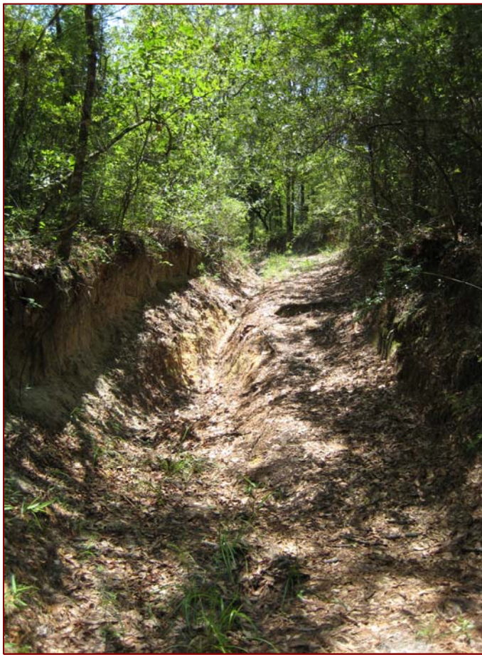
JSF Figure 2: Deep erosion requiring attention on the northern end of Road 8 on the Longbranch Tract.
