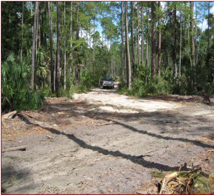
GSF Figure 1: Hard Surface Low Water Crossing combined with 2 earthen ditch plugs to restore hydrology of nearby wetland during a timber harvesting operation on Cow Creek Tract
