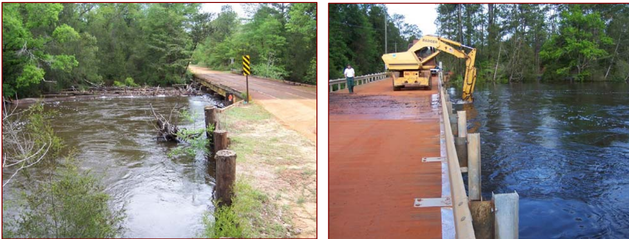
BRSF Figure 1: Pilings under the Peaden Bridge on the Blackwater River, can be weakened by debris at flood stage (L); clean-up operations like the one pictured here (R), in the spring of 2007, can prevent structural bridge problems from developing.
